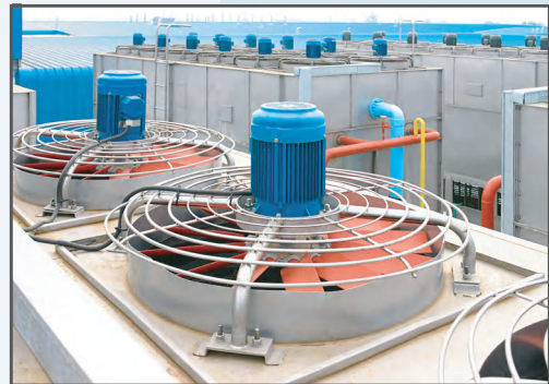
Fan and water pump
